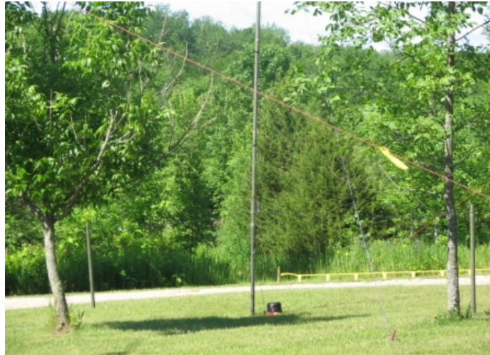
The Field Day Vertical using fiberglass telescoping mast sections. Excess coax is wound on a plastic coffee can to act as an RF choke.
